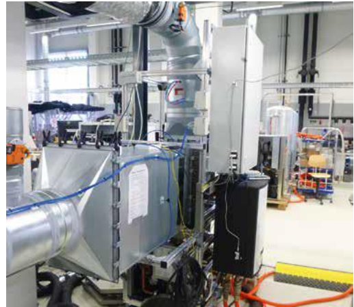
Figure 64: Setup of the demonstration unit in MOSKWA for the combined use of outside and discharged air
