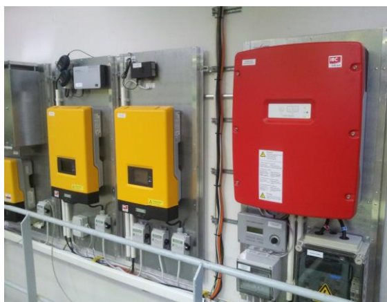
Figure 17. PV and island network inverters.
