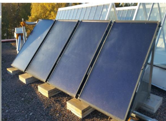
Figure 18. Flat-plate solar collectors on the roof of the K4 building.
