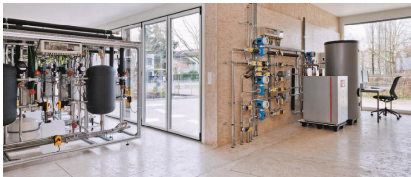
Figure 44. Second stage of the thermodynamic core (left). Heat pump and domestic hot water storage (right).
