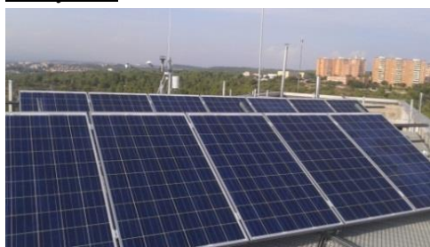
Figure 3. PV equipment on the roof of SEILAB.
