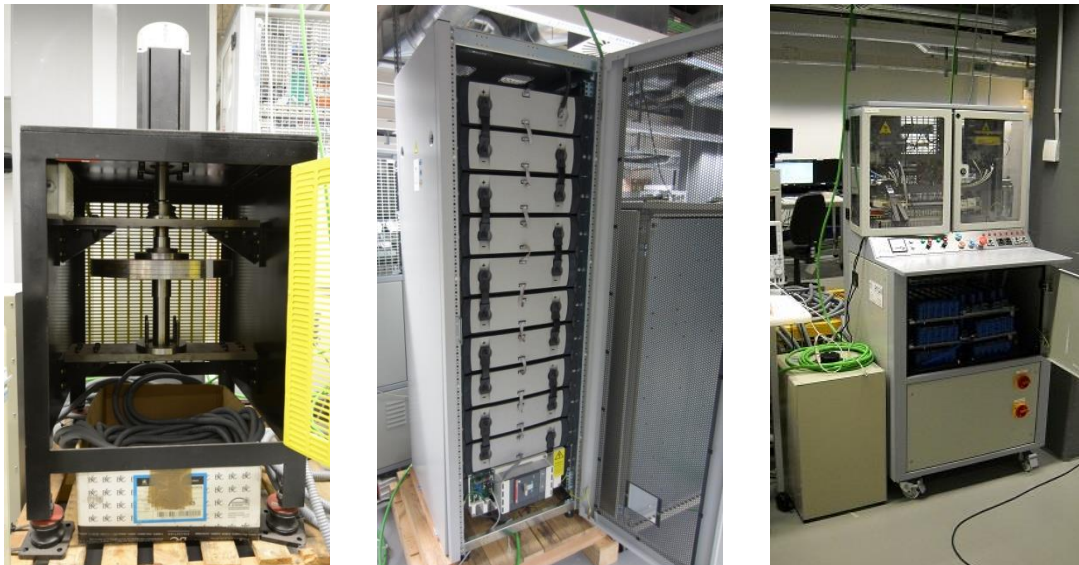
Figure 9. Energy storage systems: flywheel (left), Li-ion battery (middle) and ultracaps (right).
