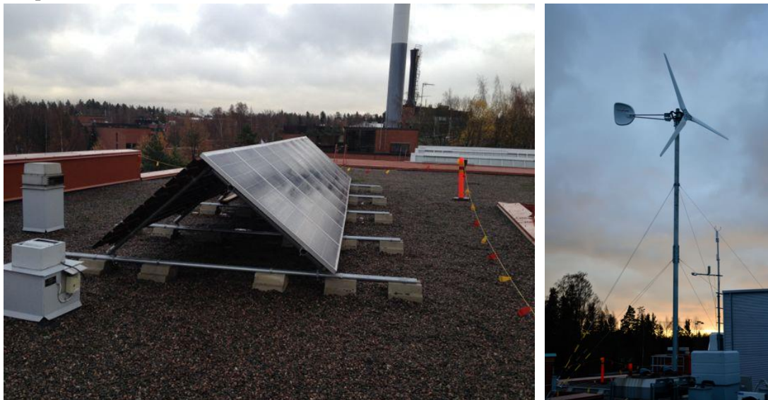
Figure 16. PV panels and microwind turbine on the roof of the K4 building.
